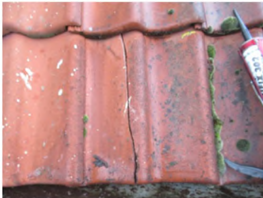
dak no. 9: gescheurde dakpan (2024)
