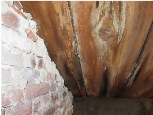
dak no. 4: lichte inrotting dakbeschot (2022)
